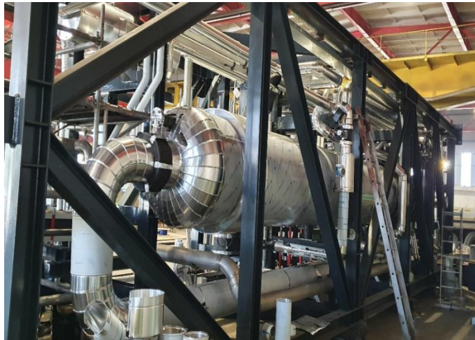
Complex steel structures - Skids, project Wloclawek Poland Client: Linde Engineering AG Period: June 2021 - Apr. 2022
